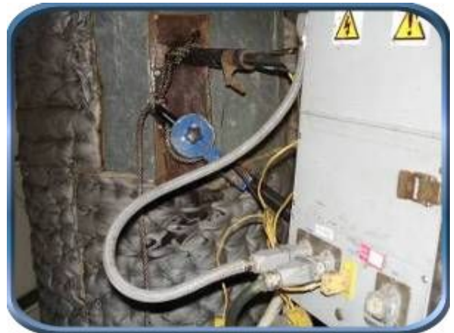
Continuous measurement probe and sample collection probe, placed in the ME4 flue.
